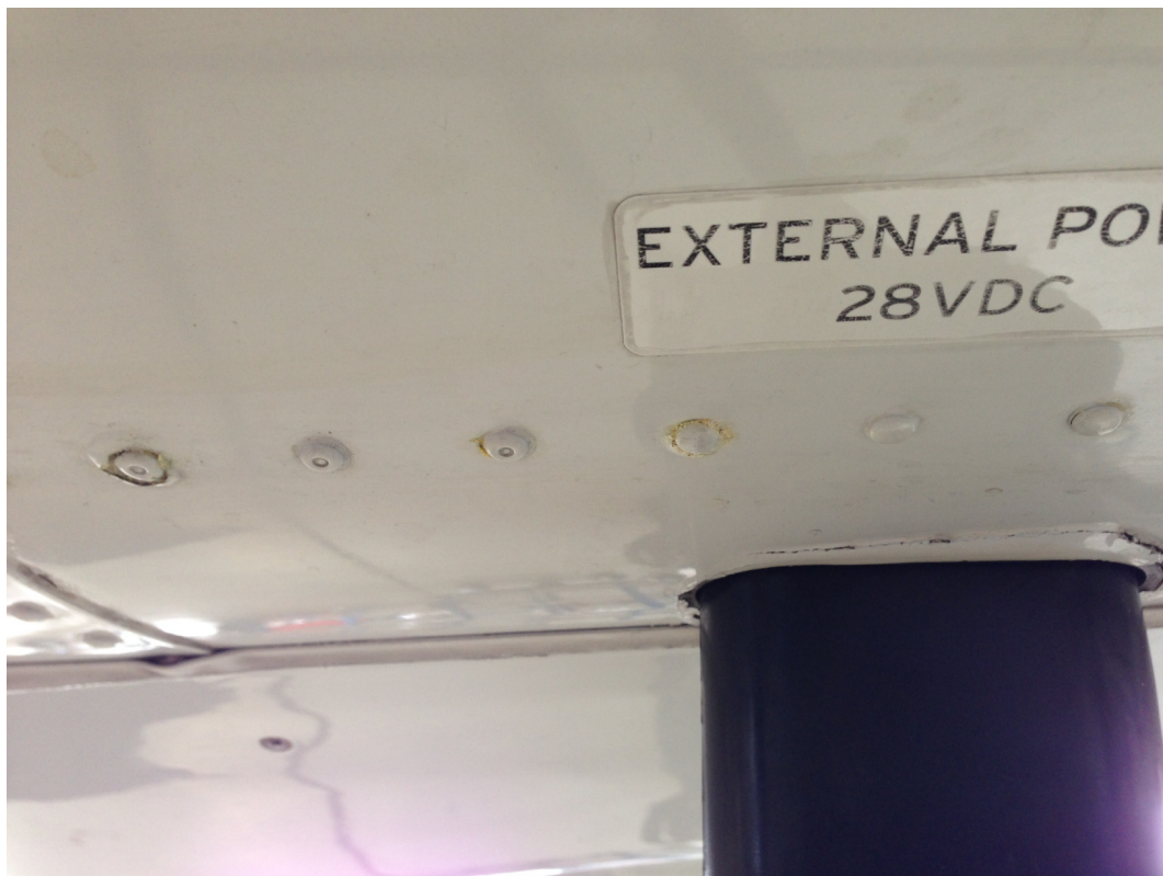
Figure 2. External Power Receptacle Rivet Corrosion
